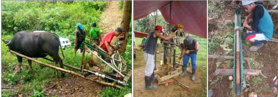
Figure 10-1. a) Mobilization of drill machine and accessories by manual hauling and at times using carabaos, b) actual drilling using YBM-YHP drilling machine, c) samples retrieval using core pusher.
